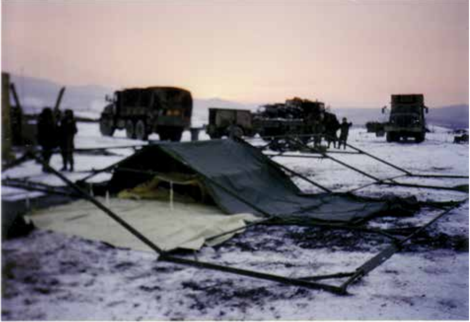
Figure 5-7. Erecting tents at Bedrock, January 1996. Photograph courtesy of Lieutenant Colonel Steven Gouge.
